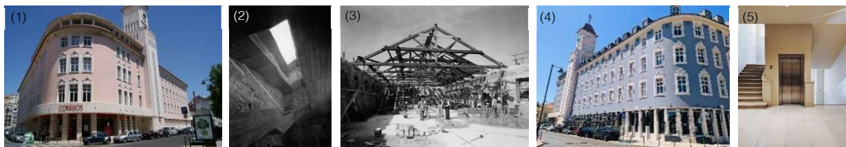
Figure 6 - (1) Corner building, before the intervention. (2) Concrete stairs, under construction. (3) Wooden roof structure, under construction. (4) Exterior facades, after intervention. (5) Clock Tower stair core, after the intervention.
